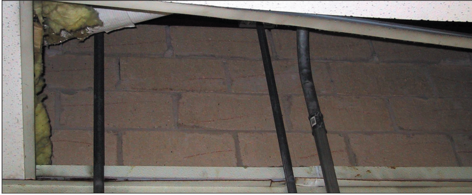
Figure 2. Typical drop ceilings may crack or be repositioned improperly, resulting in reduced contaminant control and/or increased air contamination in the plant.
