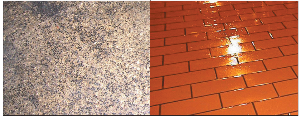
Figure 1. (Left) Plain concrete floors will spall and the exposed aggregate creates an excellent hiding place for microbes. (Right) Floor coverings should be smooth, non-absorbent and easily cleanable.
